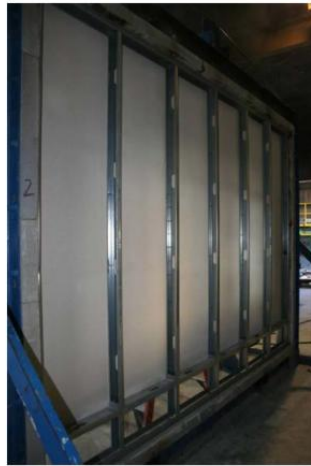
Figure B-1. Base Wall Layout with One Layer of Magnum ® Board Installed.
